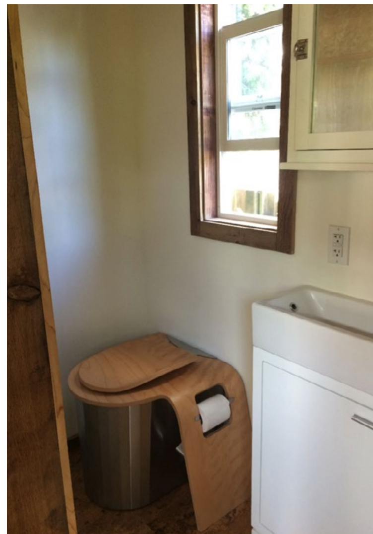
An Ecodomeo urine diverting compost toilet in a tiny house.
